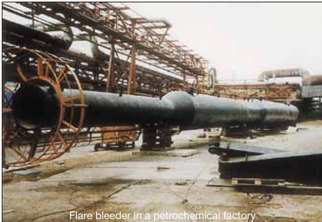
Flare bleeder in a petrochemical factory
