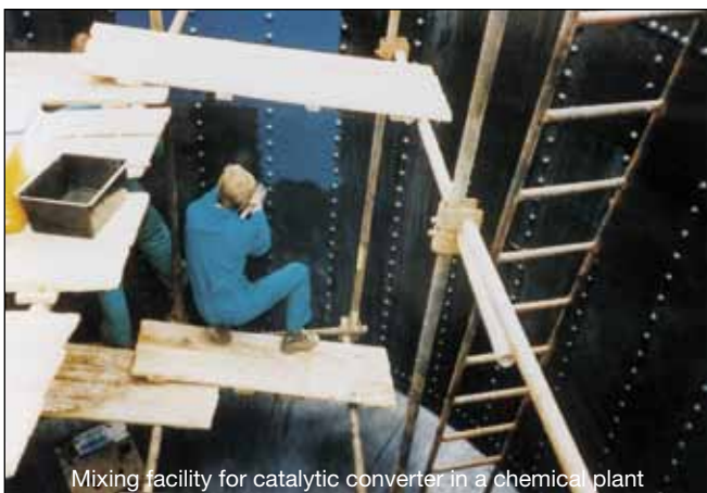
Mixing facility for catalytic converter in a chemical plant
